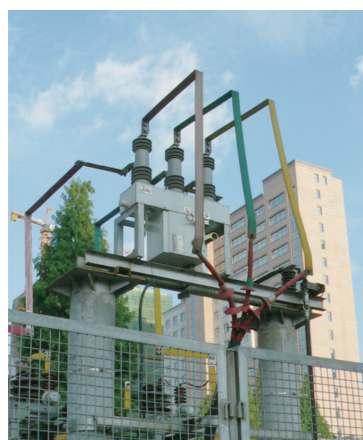
热缩终端运行图 Heat-shrink Termination Service Photograph
