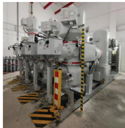
GIS终端现场运行图 GIS Terminal On-site Operation Photo
