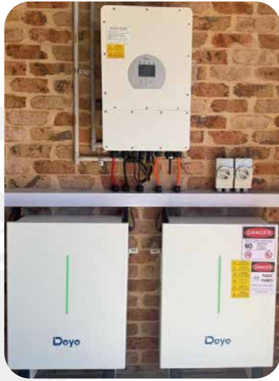
► Inverter: 3Ph 10kW SUN-10K-SG04LP3-AU ► Battery: 10kWh RW-F10.2*2 (pcs)
