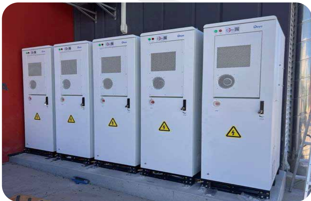
► Inverter: 3Ph 250kW SUN-50K-SG01HP3-AU*5 ► Battery: 300kWh GE-F60*5 (pcs)
